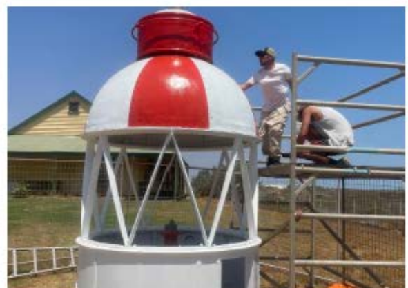
Pictured: Workers have almost completed the lighthouse as part of the Carnarvon Heritage Precinct Revitalisation.
